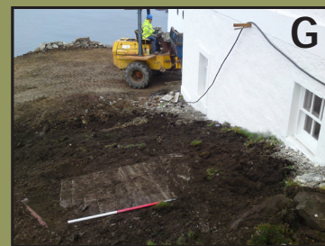
A former air raid shelter blast wall was discovered during groundworks when the site was renovated in 2012-14.
